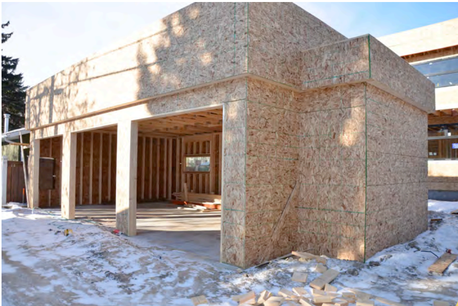
Detached Garage - where the secondary suite is supposed to be on top of.
